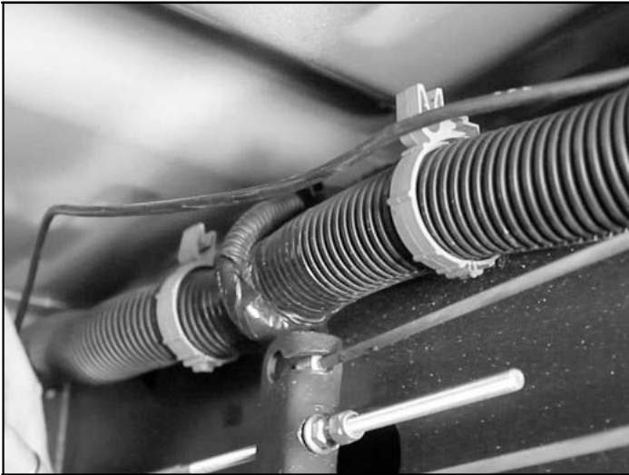
Route harness 250-8550 to the front driver side of the truck attaching it to the factory harness with cable ties.
